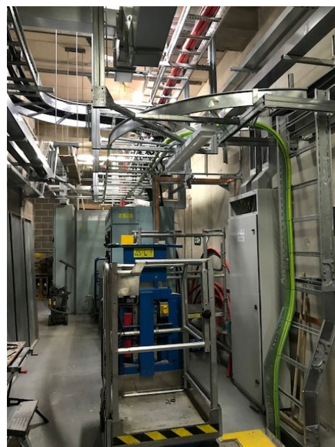
Fig.2 Fit out and commissioning of one of the electrical rooms below ground
